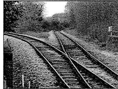
Last year a survey found the rail bed and structures were sound
